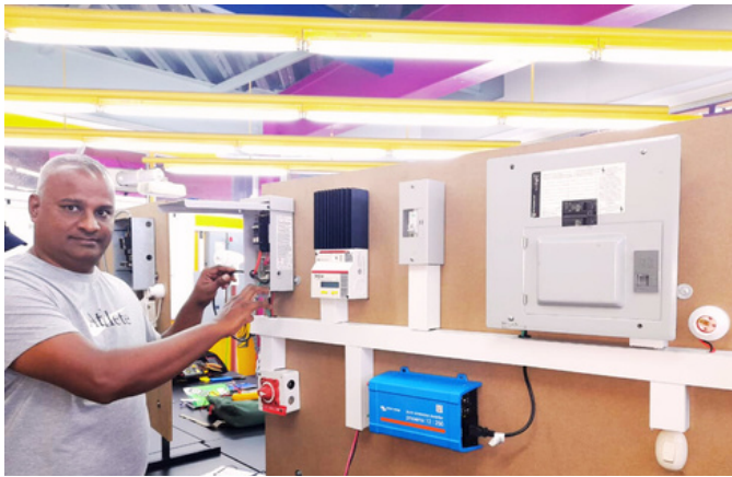
Michael Mandole - Automation Service Technician IMPLEMENTING SOLAR POWER SYSTEMS FOR POWER GENERATION: PHOTOVOLTAIC INSTALLER Level 1
