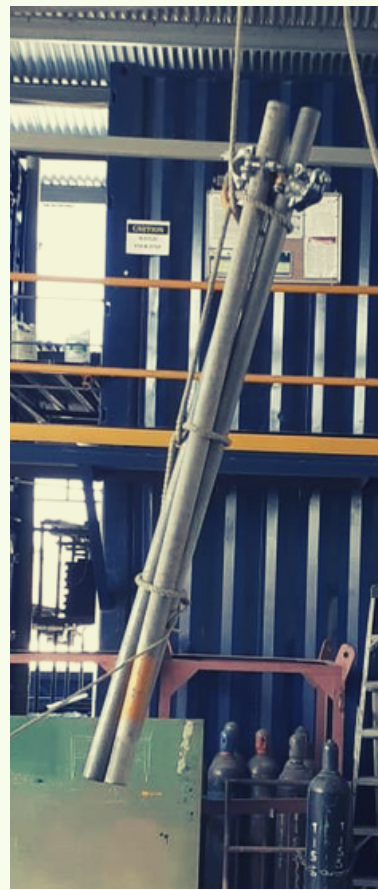
Figure 2: Proper tie that should be used to lower pipes (lasso tie with multiple slip knots as required). A tagline should also be used to guide the load
