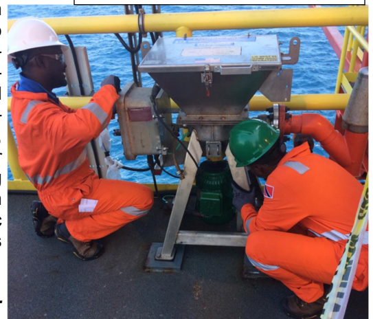
Installation of a Tuff Gut macerator on Mahogany B that was repaired in the TOSL machine shop.
