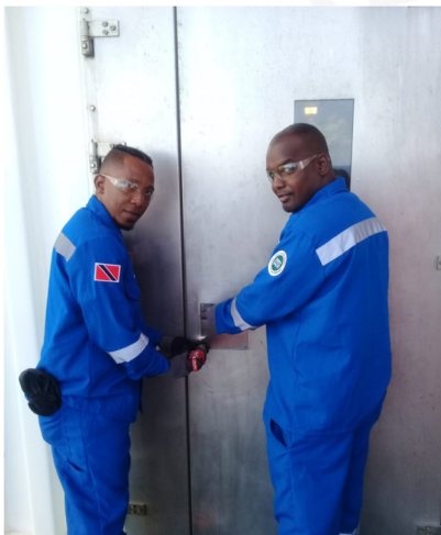
Preventative Maintenance being completed on a walk-in chiller in the galley area on Mahogany B
